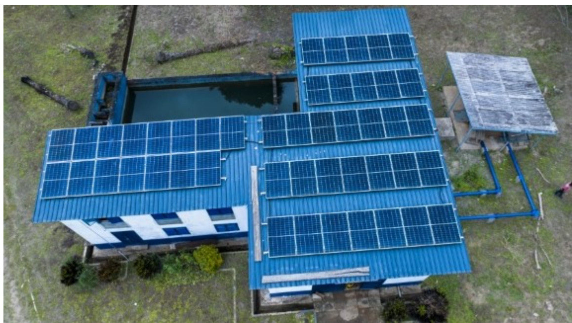
1. Aerial view of Likpe Community Water Pumping Station © GIZ
