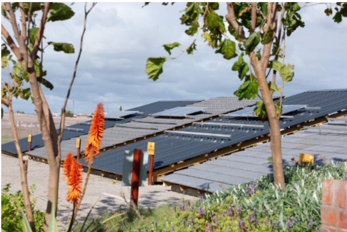
PV Panels on rooftop ©GIZ/Jesse David Preyser
