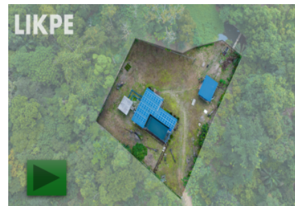
Installed solar panels on the Likpe Community Water Pumping Station © GIZ
