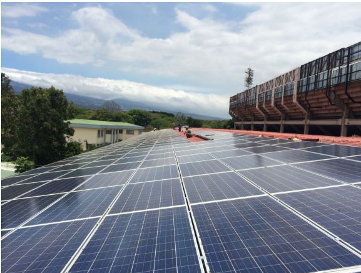
Integrating Solar Power in to the West African Power Pool for enhanced grid stability © GIZ
