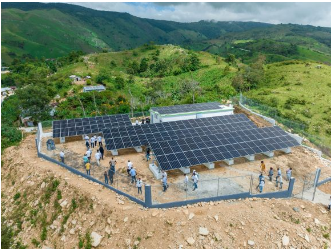
Panoramic view of the photovoltaic plant for the rural community in Sabana Real, Dominican Republic © GIZ (Energy Transition Project)
