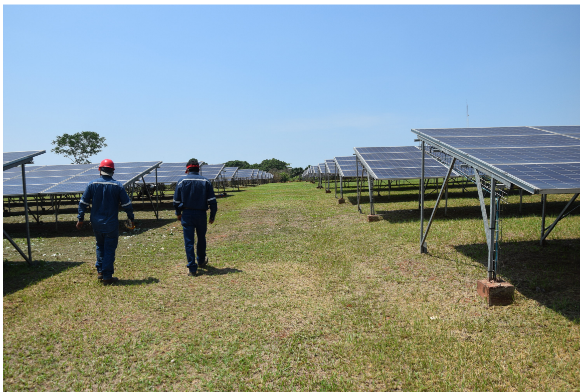
Photovoltaic Solar Plant. Cobija, Bolivia. ©PEERR/GIZ
