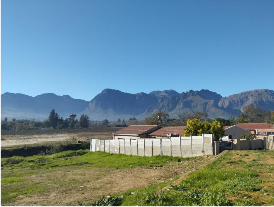
Part E Chapter 3 Image 3. The eroded embankments pose a safety risk to the stability of residential development close by.
