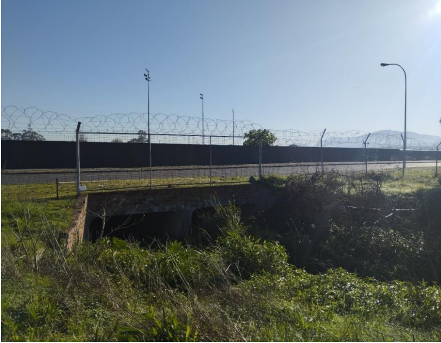
Part D Chapter 4 Image 3. The Boontjies River exits a large culvert to flow beneath Bo-Dal Josafat Street before exposure in the Dal Josafat Stadium.
