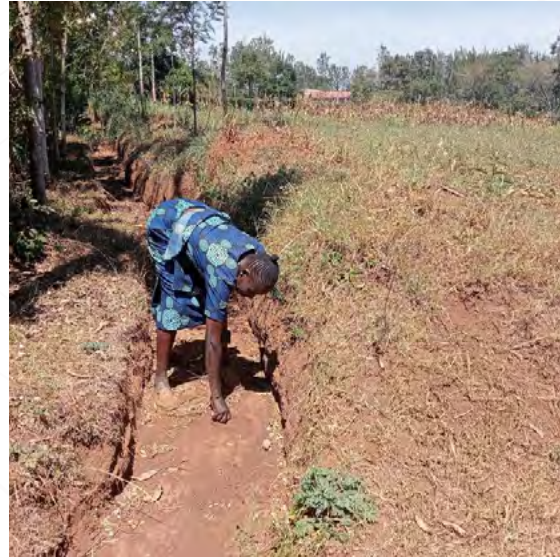
Silt accumulation in a retention ditch (William Akwany)
