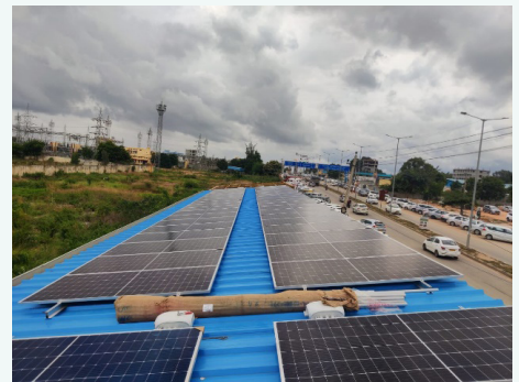
Picture of Solar PV panel installed in the rooftop Photo Credit : GIZ
