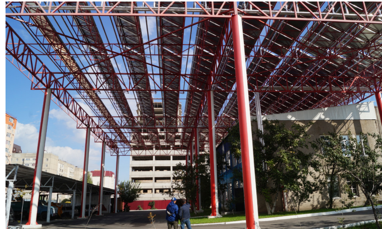
1,75 MW Solar water pre-heating installation for rotor boiler house in Bishkek, Kyrgyzstan. 2024
