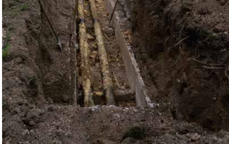
Worn-out infrastructure in Zviahel: pipes for transporting heat to homes. Modernisation is urgently needed.
