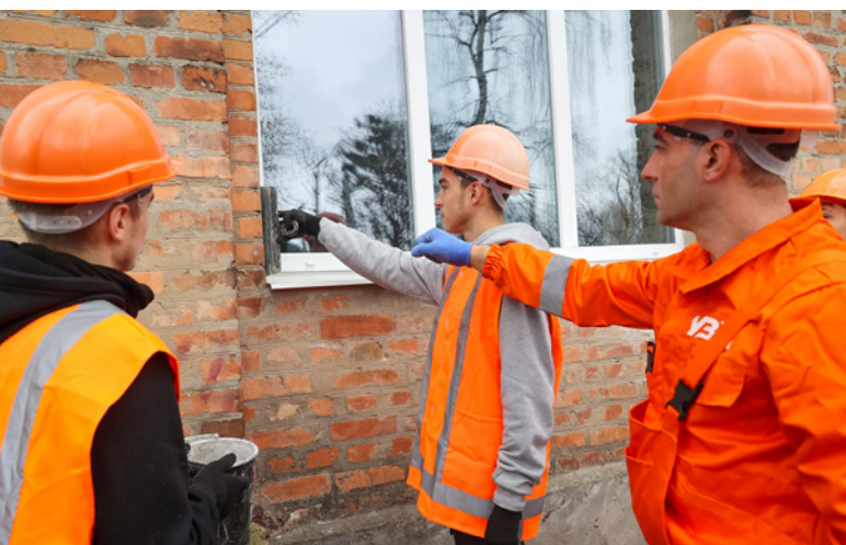
Build back better: Vocational school students in Kharkiv learn how to install energy-efficient windows in the war-damaged school building.
