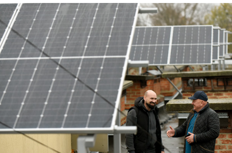
Energy security: Thanks to the photovoltaic system on the roof, a children's hospital close to the front line can look after its patients even during power cuts.
