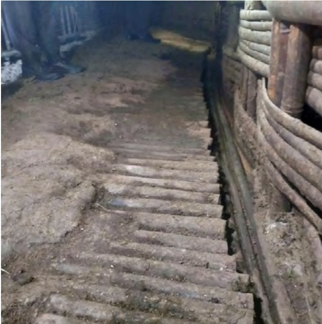
The floor of the cattle stall drains the urine straight to the collection chamber set outside the house. (Gerba Leta)
