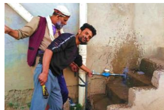
Installation and replacement of damaged water meters in Dhamar Water Utility to reduce nonrevenue water.
