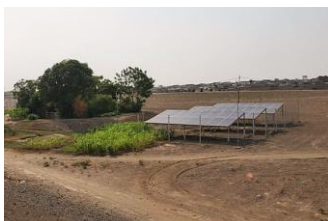
Installation of solar water pumping systems to maintain the water supply services in Zabid Water Utility, to improve resilience and reduce the running costs.
