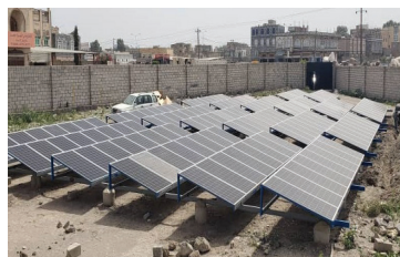
Installation of solar water pumping system as a project in selected LCs to mitigate financial hardship and enhance the reliability of water supplies.
