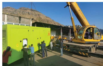
Replacement and maintenance of electric generators, pumps and vehicles to maintain the water production and supply.
