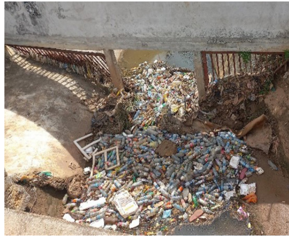
A storm water drain in Lusaka blocked with waste.
