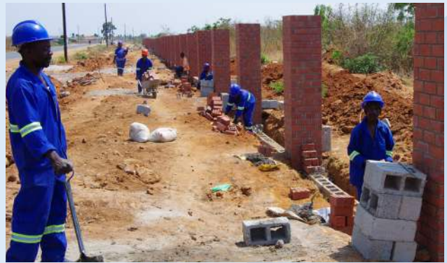
Preventing the encroachment of the Wellfield Shaft 5 in Lusaka by protecting it through a fence.
