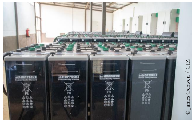
Photo: Battery Energy Storage
