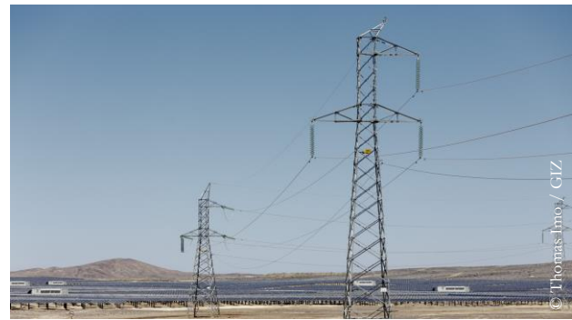
Photo: Power Poles with PV in the background
