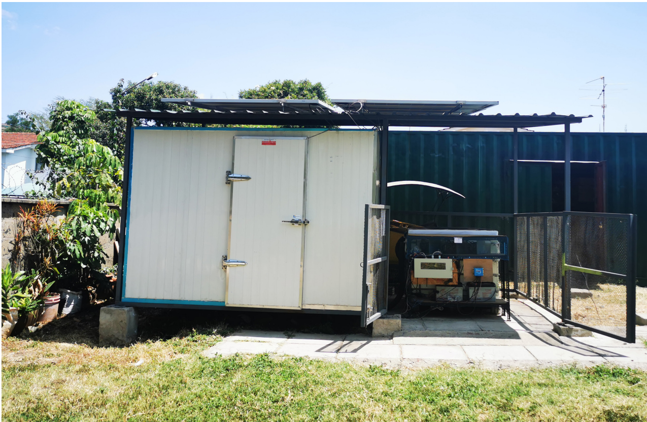
Picture 7. A photovoltaic-driven walk-in cold room container in Kenya.
