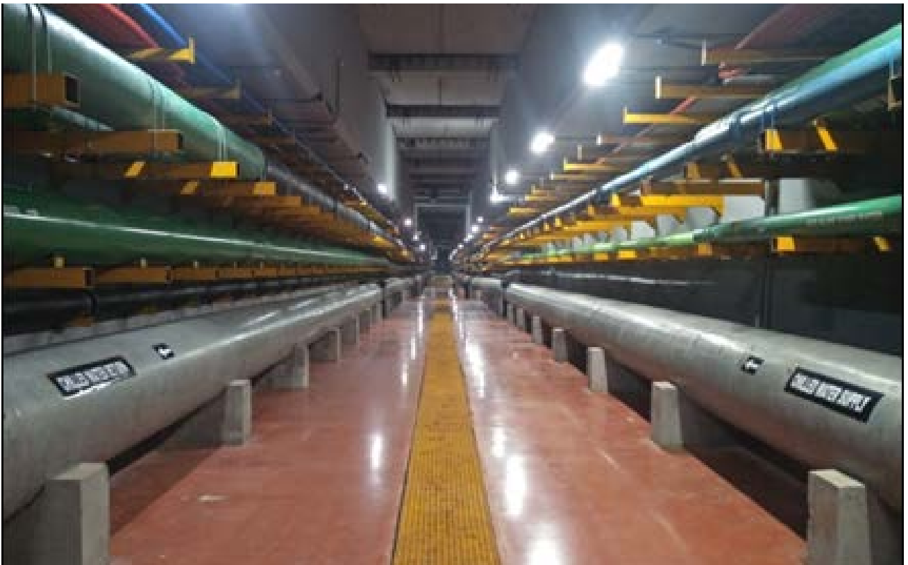
Figure 25: GIFT City DCS: View of DC System Piping Network in Utility Tunnel
